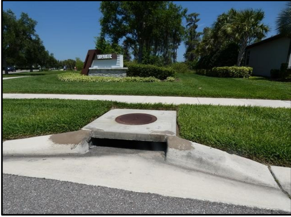
Stormwater Drainage Curb Inlet
